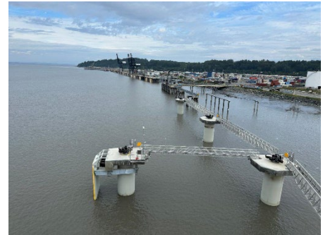
Tidal challenges and silty ground present design challenges. A million cubic yards of silt need to be dredged per year from this area.
