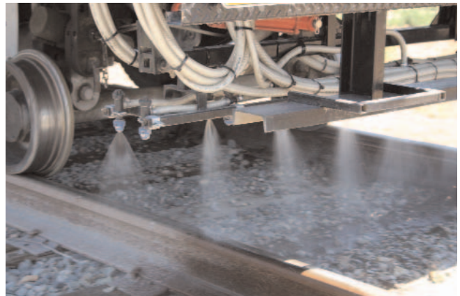
A specially-equipped truck directs weed control products directly at the track bed.
