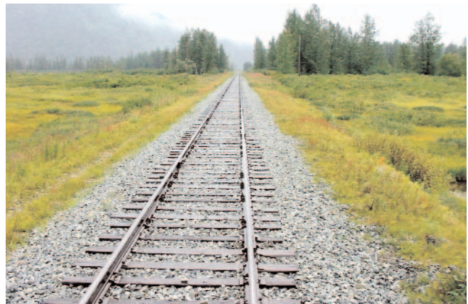
Optimally, the Alaska Railroad track would be free of weeds, providing an uncompromised platform for train movement.
