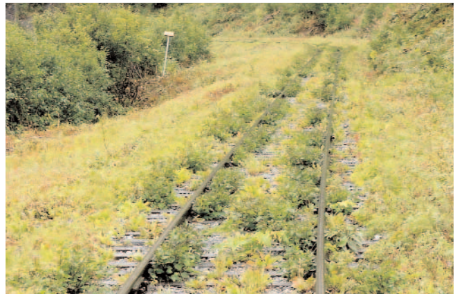
Overgrown weeds on the track bed are nearly impossible to get rid of with non-chemical methods.
