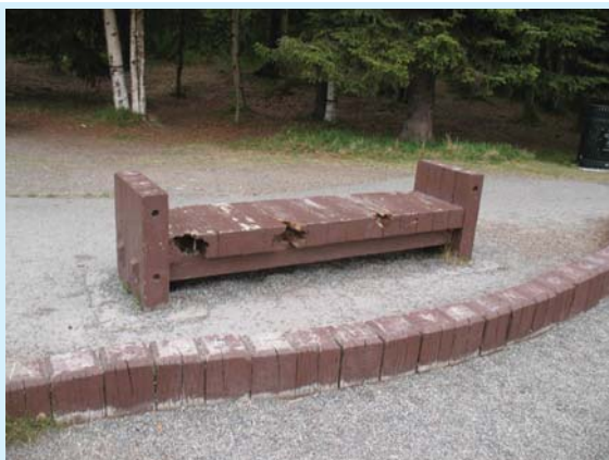
The damage done to this bench in the upper playground area exceeds the Limits of Acceptable Change (LAC) and should be replaced or repaired.
